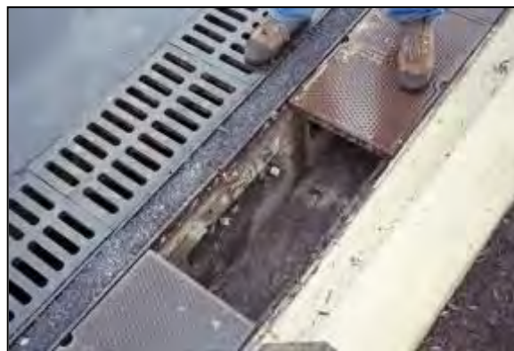
Perimeter Sand Filter
