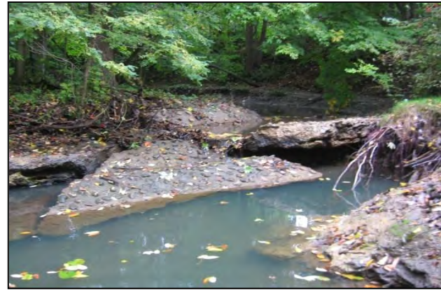
Existing Infrastructure Blocking Fish Passage (Source: Baxter & Woodman, Inc.)
