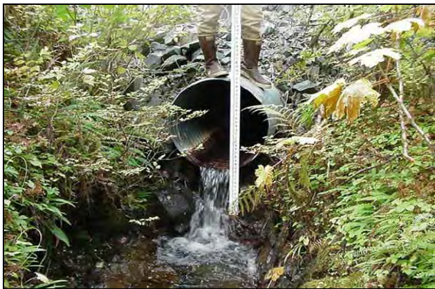
Culvert Blocking Fish Passage
